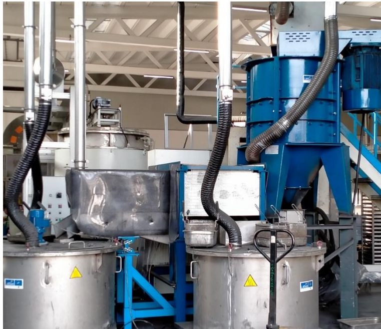
Overview of the mechanical section
