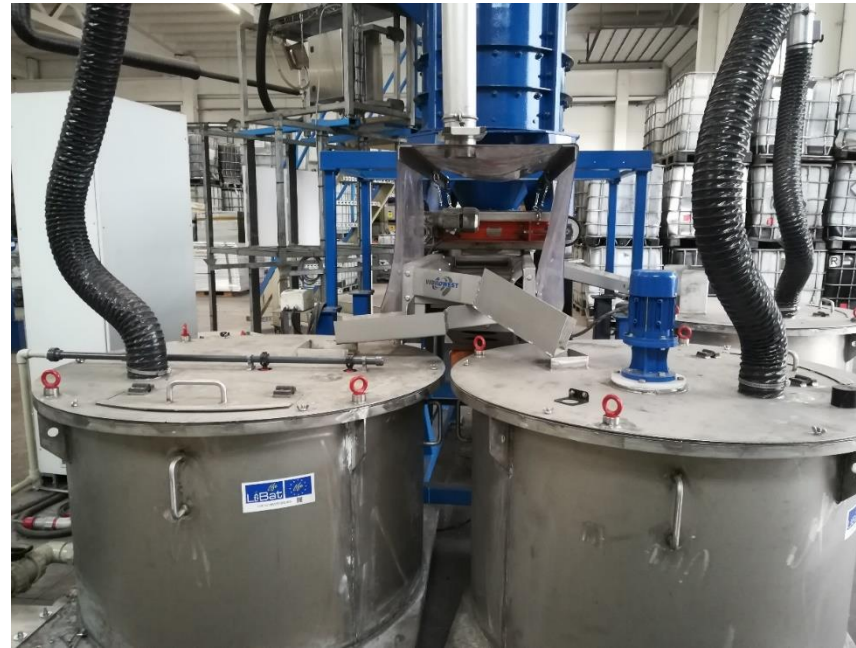
Mechanical section and neutralization reactors
